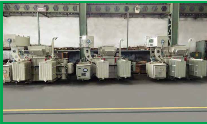
Transformer on floor.
